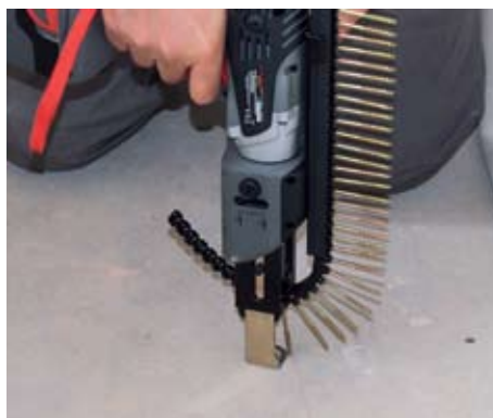
▲ Pic.4 Screws are easily driven in. Chipboard flooring is an ideal application
